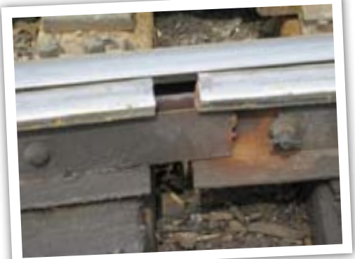
Trainees discovered a broken switch point in Burnaham Yard during their first day of field training.
