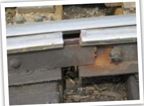
Trainees discovered a broken switch point in Burnaham Yard during their first day of field training.
