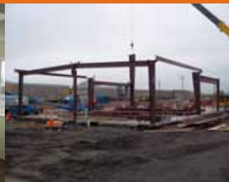
Iron workers erect steel framing on the new Gibson Yard building Dec. 20.
