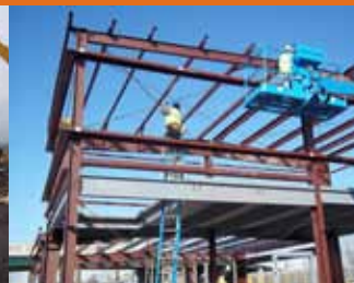
Iron workers erect steel framing on the second floor of the Gibson Yard building Dec. 29.
