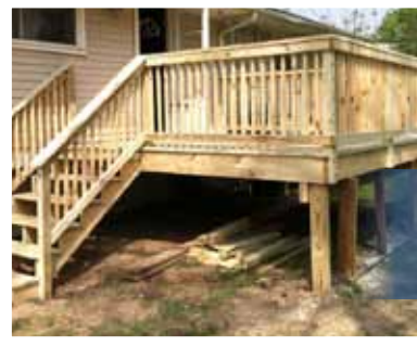
Railroaders made a colleague's summer more enjoyable and comfortable by building a deck during a weekend in May. IHB supplied funding for material.
