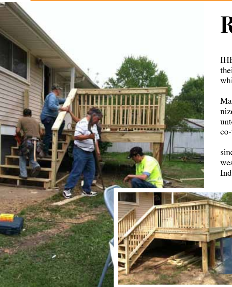
Railroaders made a colleague's summer more enjoyable and comfortable by building a deck during a weekend in May. IHB supplied funding for material.
